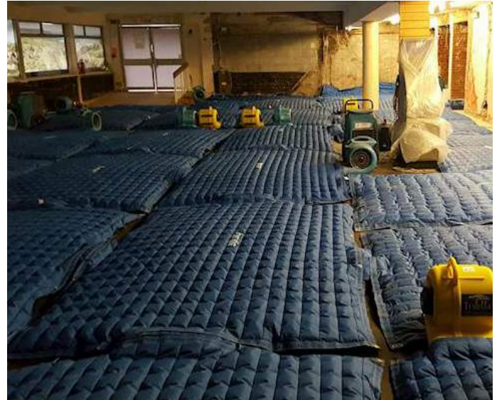
Heat mats and dehumidifiers installed in the flood affected shop
